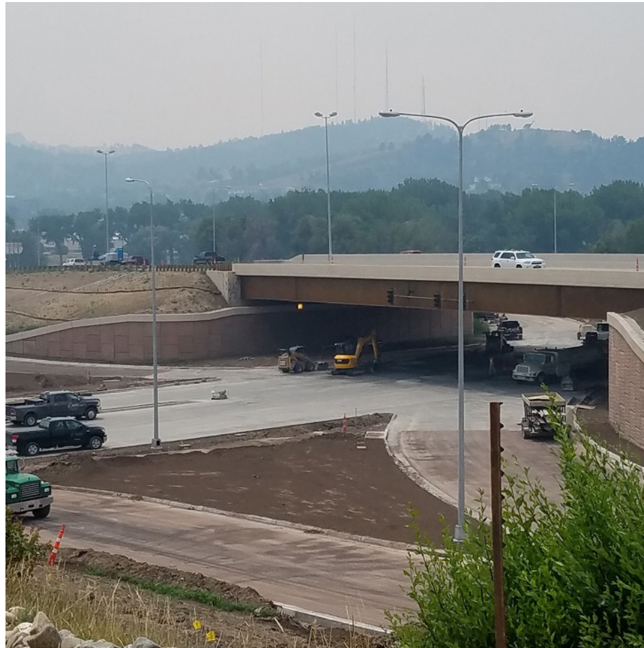
North Street beneath the bridge, and ramps to Central High School and to the I-190 north bound lanes is nearing completion.
