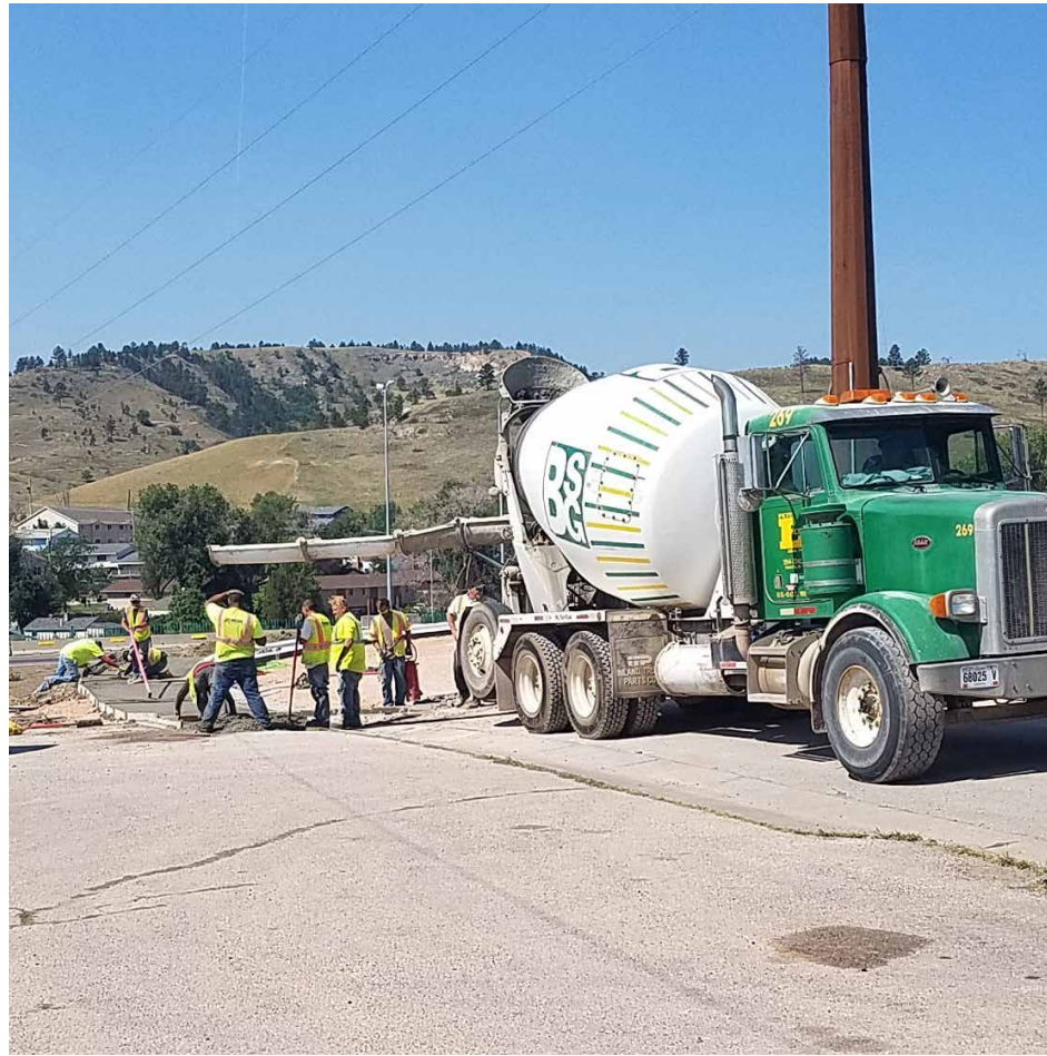
Curb, gutter and sidewalk was poured along West Boulevard North in preparation for final paving of the street.
