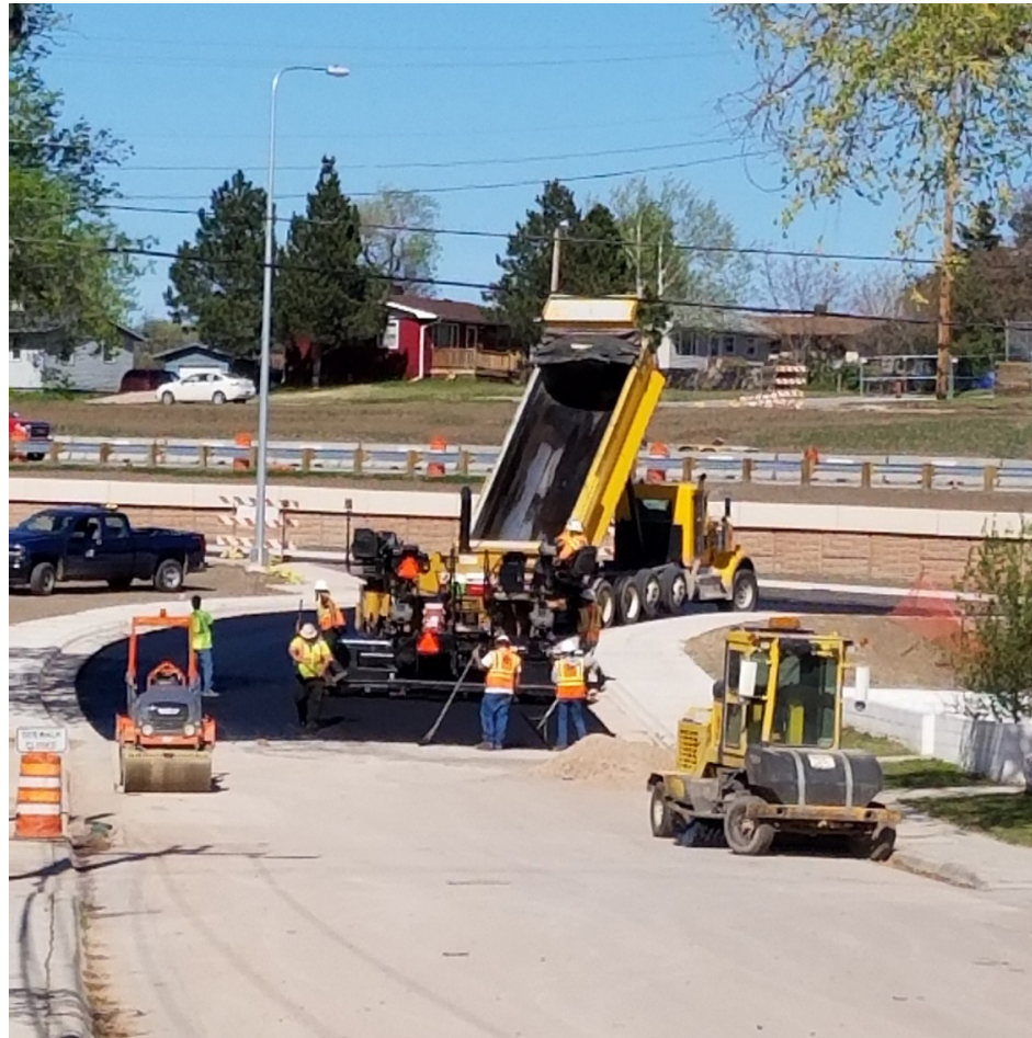
Asphalt crews have been working in the Silver Street neighborhood area west of I-190 to complete street improvements.
